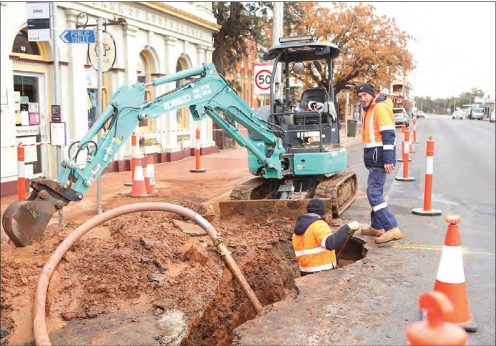
• The burst water main on Donald's main street receiving attention from GWM.
